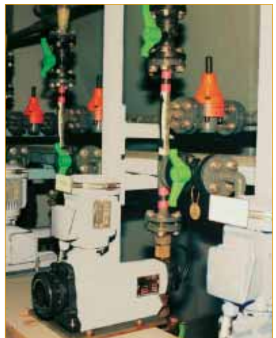
Ferric chloride pumping in purification station
